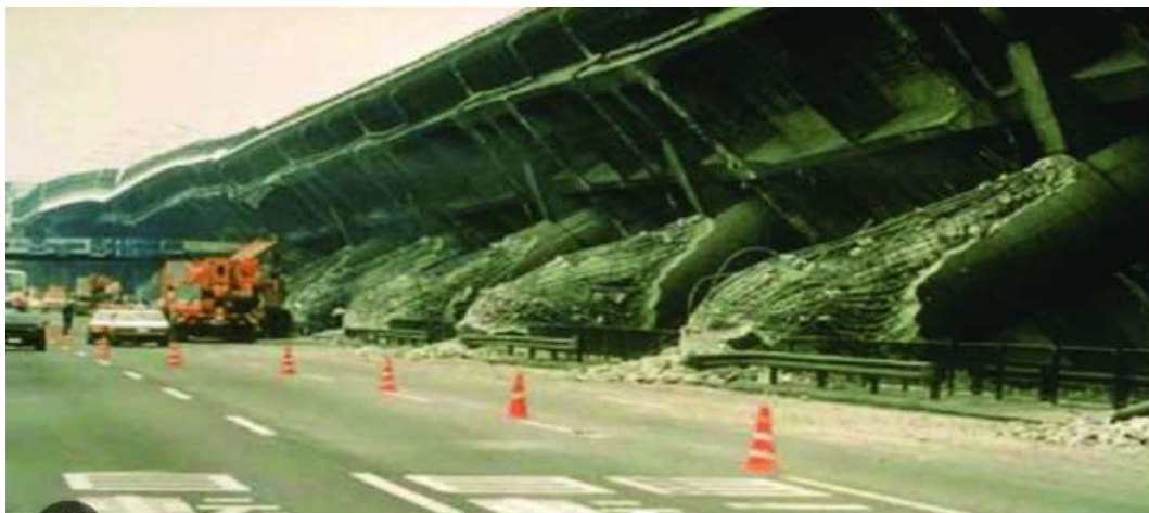
3-rasm. 1995-yil Hyoge – Ken Nanbudagi zilzila. Xigashi-Nada viaduki
