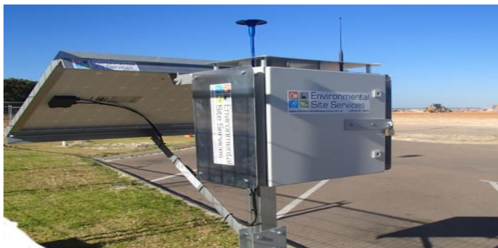
Figure 2. Air Quality Monitoring Station
